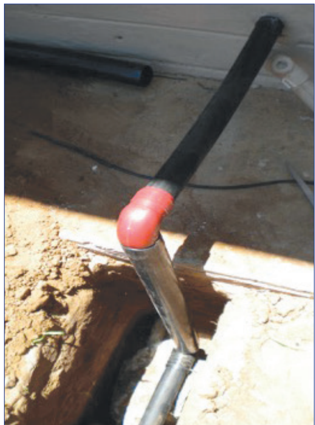
FIGURE 2: Grey water system in Omaheke region (piloted by DRFN)
